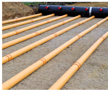
Ground-air heat exchanger
